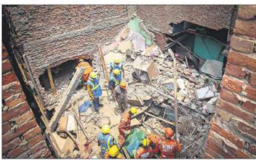
Emergency responders carry out rescue operations after a building collapsed at Janta Colony, in the Wazirpur area of Delhi on Saturday.
